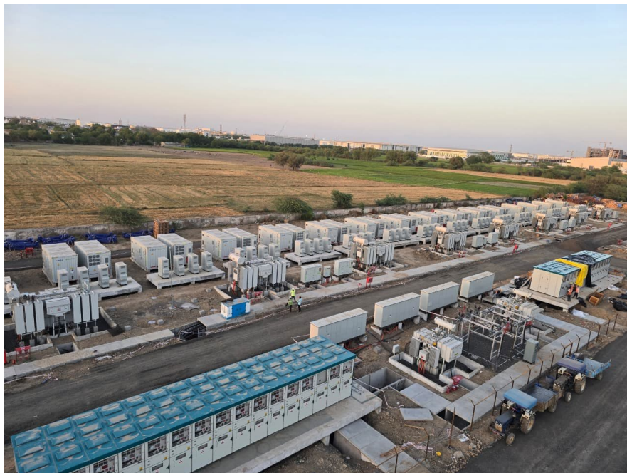
IndiGrid's 180 MW / 360 MWh BESS Project – Gujarat BESS Private Limited (GBPL)
