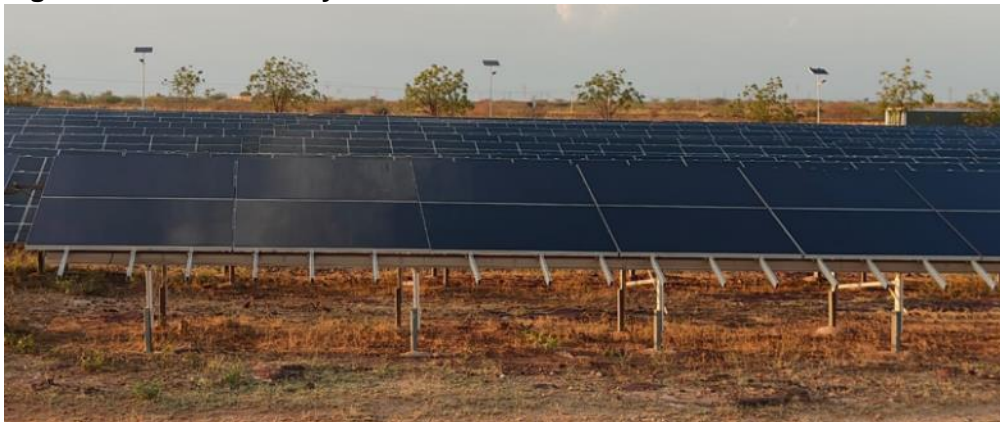
Figure 75: Solar PV array
