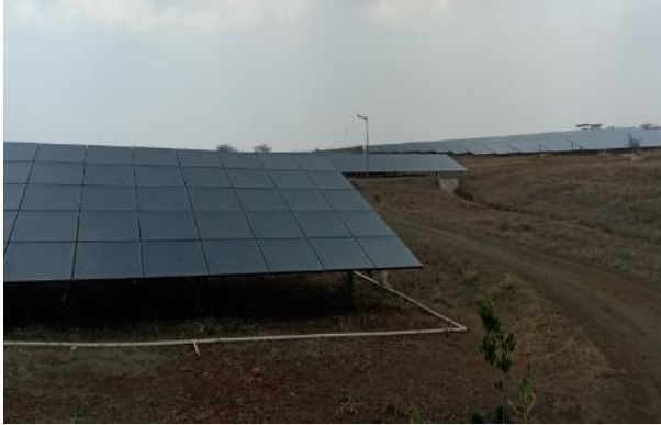
Figure 25: Solar PV array
