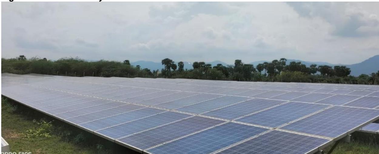
Figure 38: Solar PV Array
