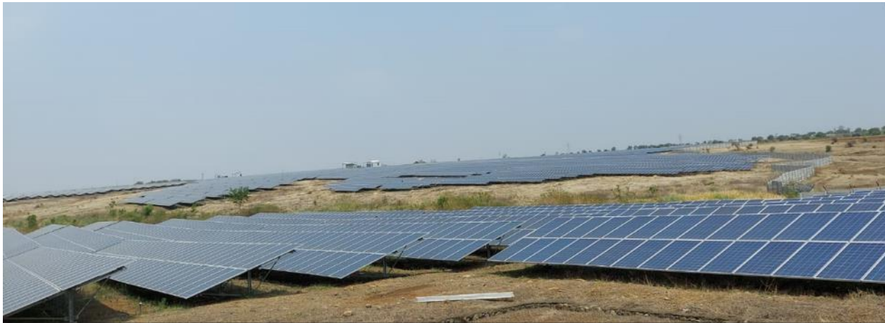
Figure 17: Solar PV Array
