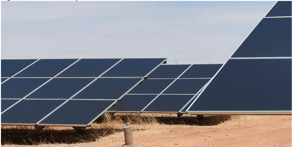
Figure 78: Solar PV array
