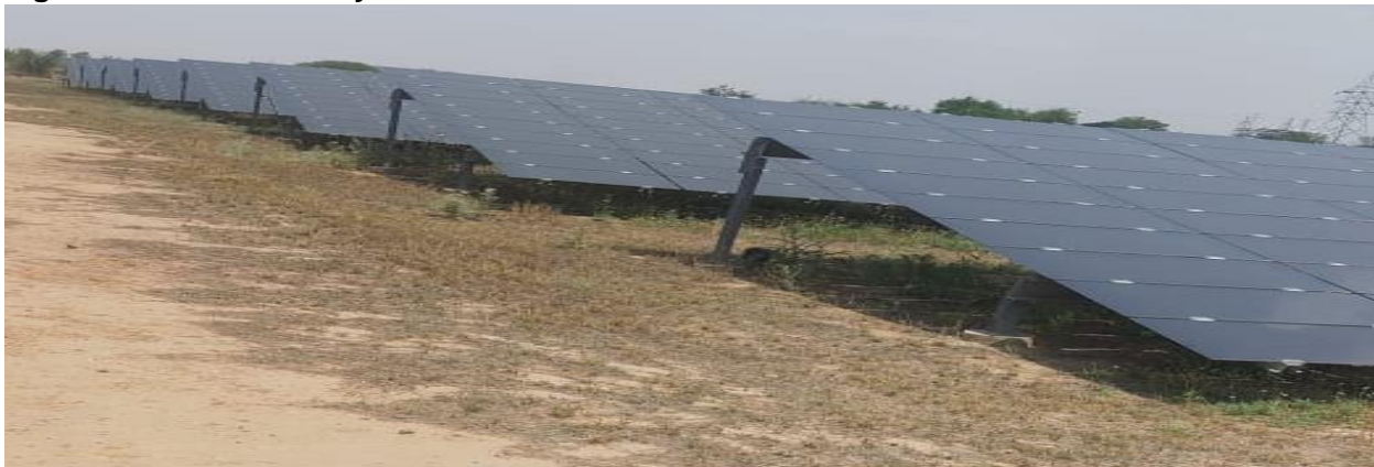
Figure 72: Solar PV array
