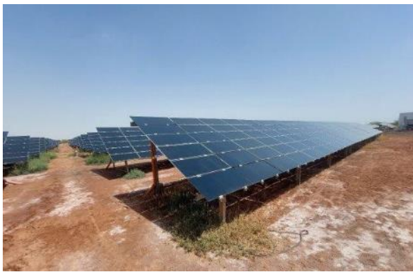
Figure 11: Solar PV array
