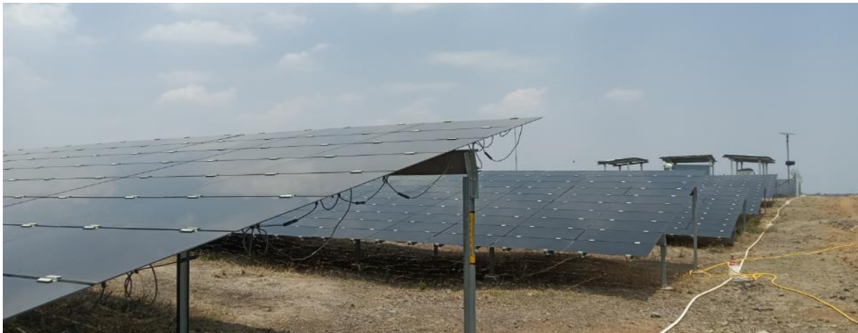
Figure 30: Solar PV Array
